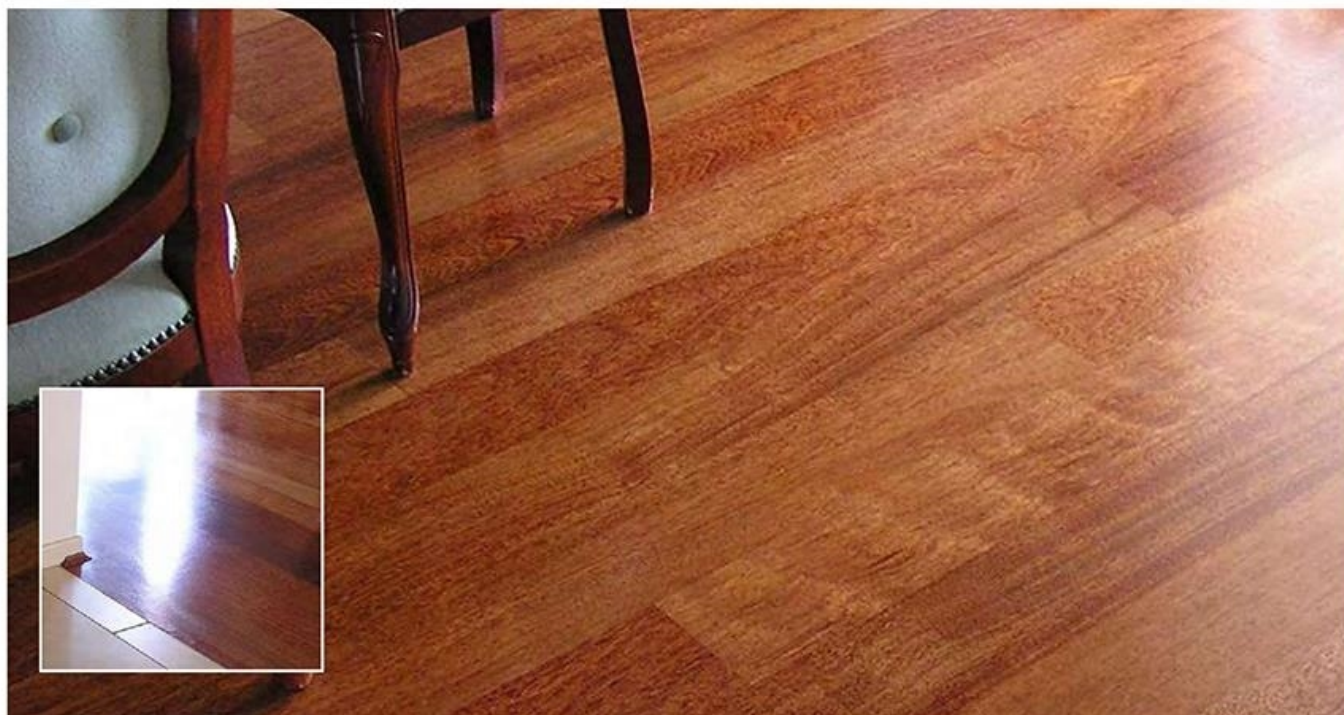
When site sanded and finished minor finishing imperfections are acceptable.
