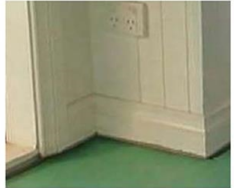
Underlay is cut neatly around corners although it is recommended to have it raised at walls to at least the height of the floor.
