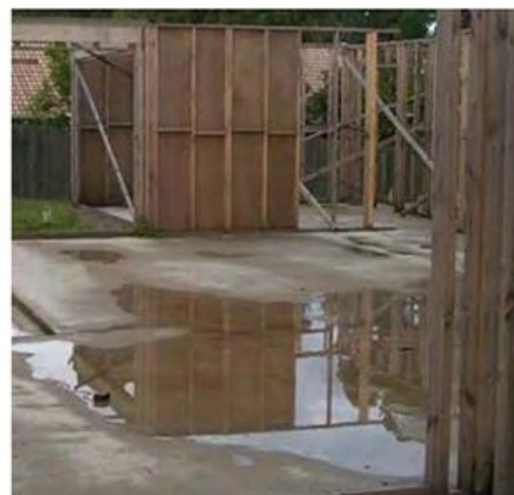
The puddles indicate low areas in this slab
