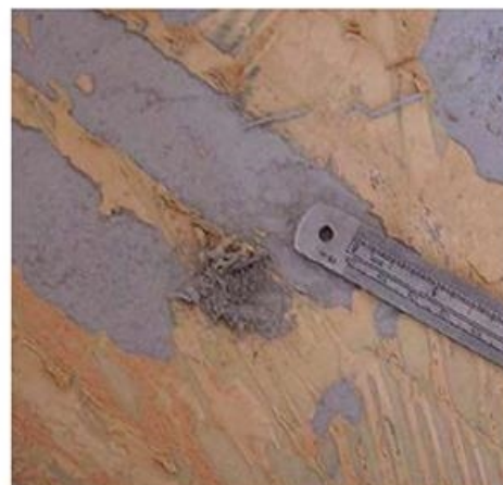
Leveling compound with insufficient strength
